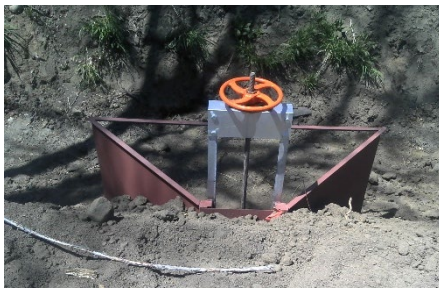
water control device
